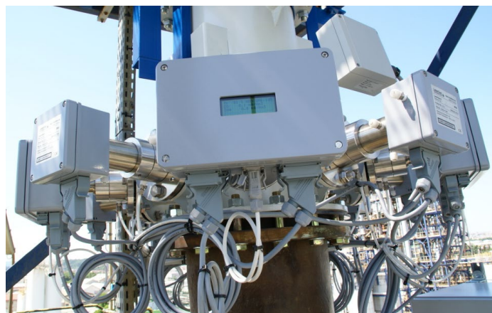
Figure 1: Five TDLAS analyzers mounted on a stack.
