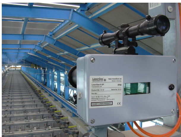
Figure 3. Fence-line monitoring using an open path TDLAS instrument.
